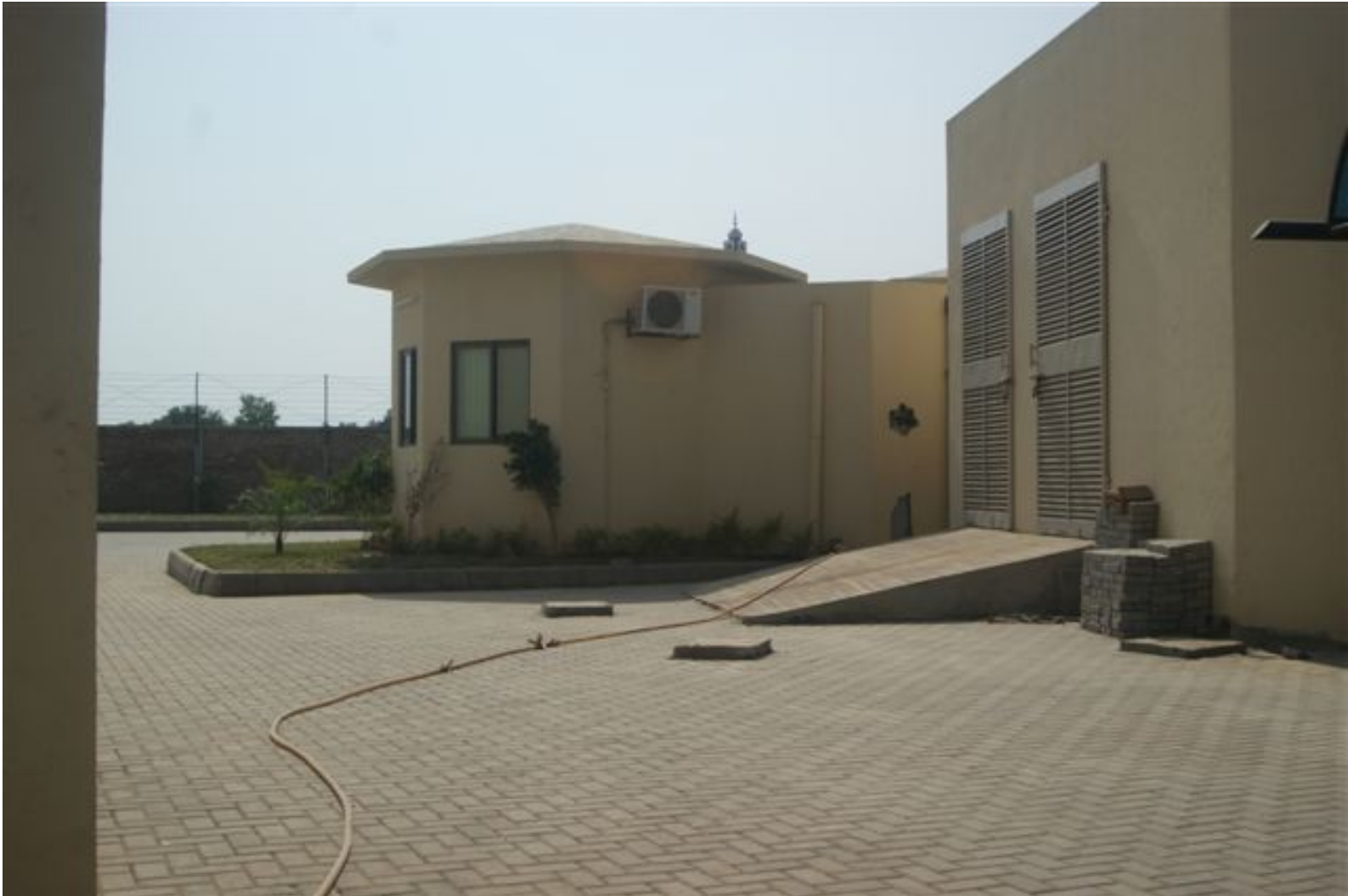
Generator View and Rear View of Gate office
